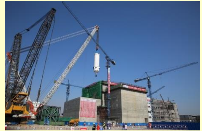
Small Modular Reactor HTR-PM at China
